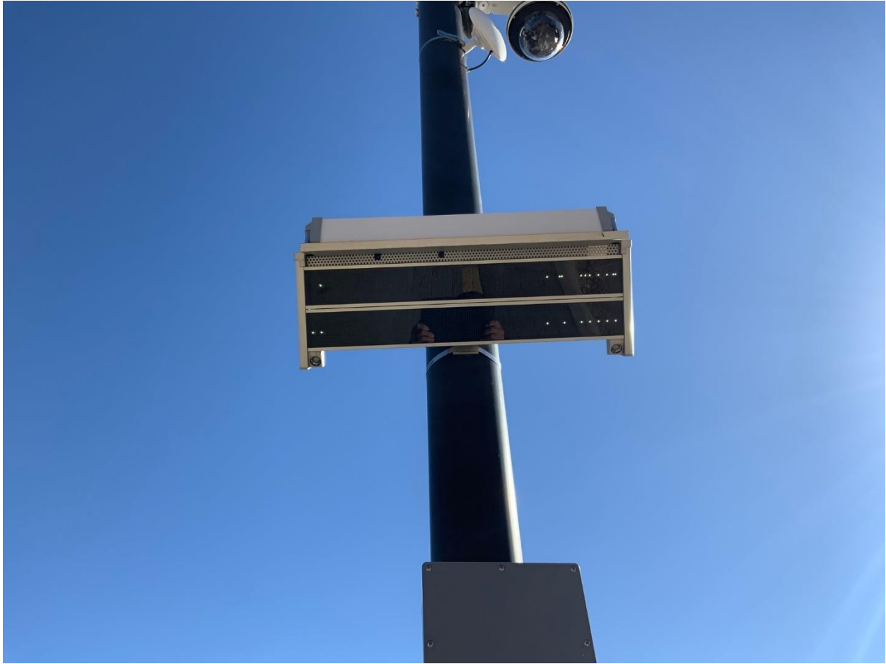
Quincy Street Station North Side Solar Powered DMS 3 of 3.
