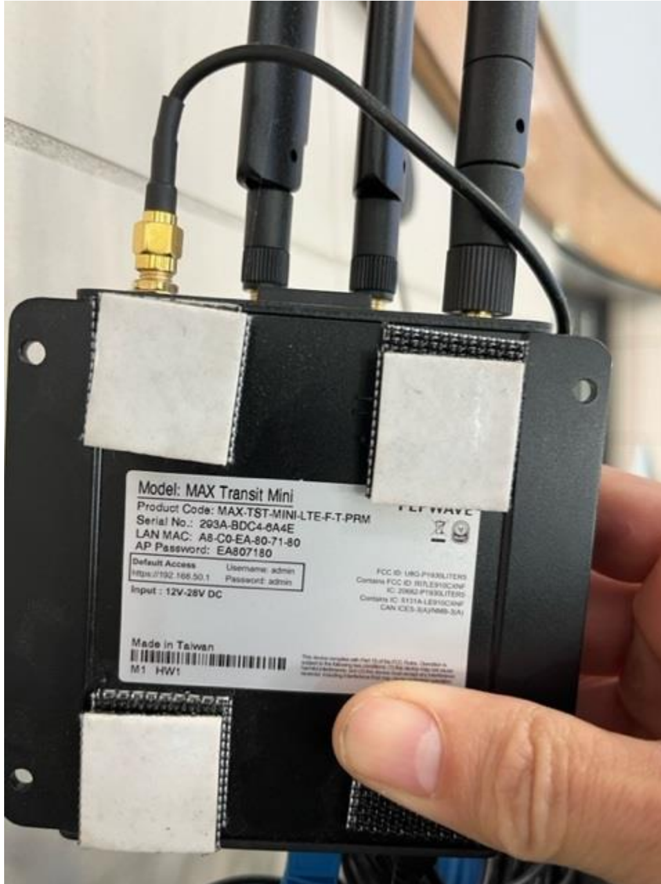
Cellular Router at Quincy Street Station
